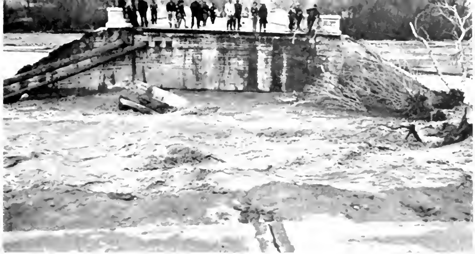
Approach to Castaic Creek Bridge on U. S. 99 in Los Angeles County washed away
